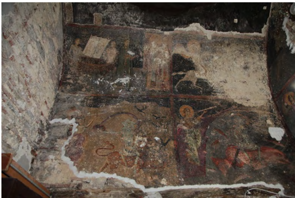
III. 113. Church of St. Demetrius in Veles, frescoes on the northern wall of the narthex (1297). Photo: S.V. Maltseva
