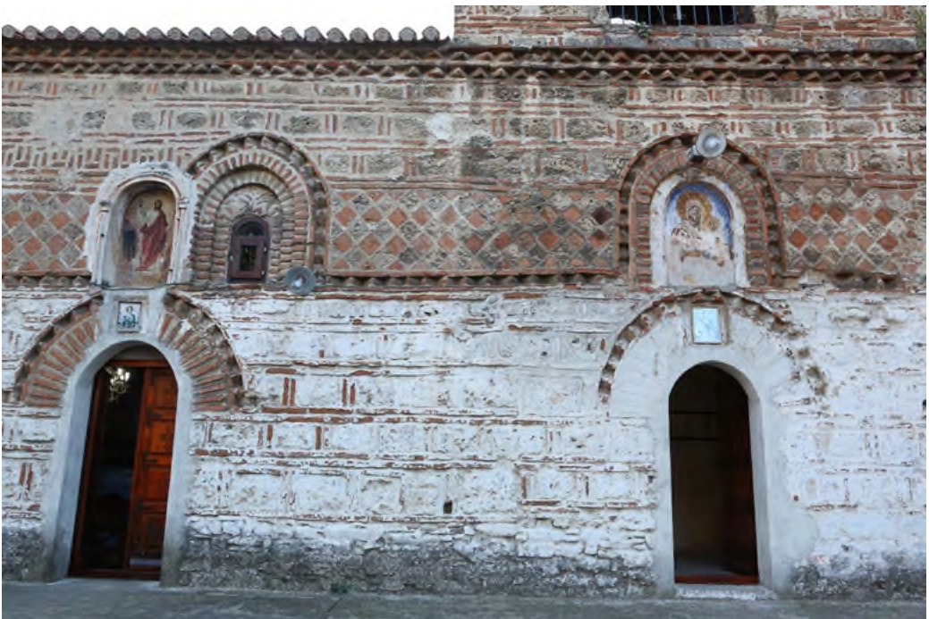
III. 122. Church of St. Demetrius in Veles, northern facade (1297). Photo: S.V. Maltseva
